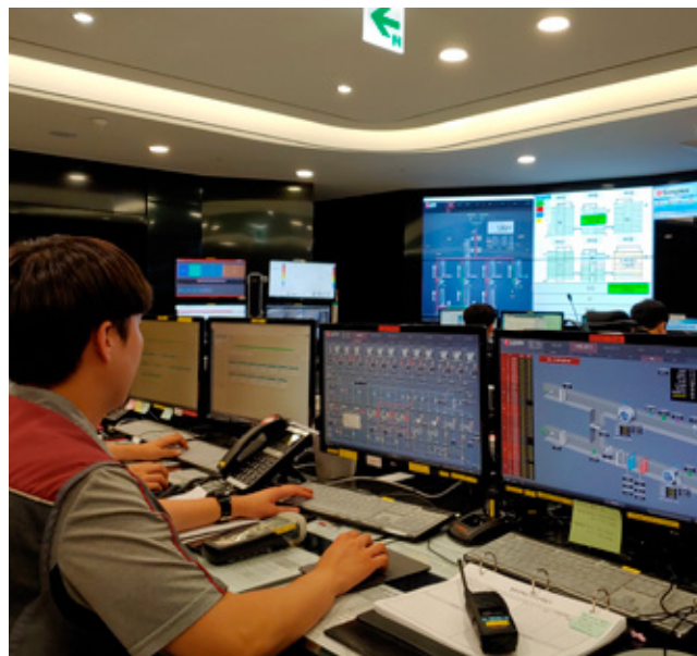
LG Science Park Control Center equipped with a solution for integrated building controls and energy management
