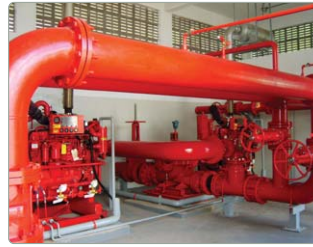
Overseas EESH technical support - pump facility (Brazil)
